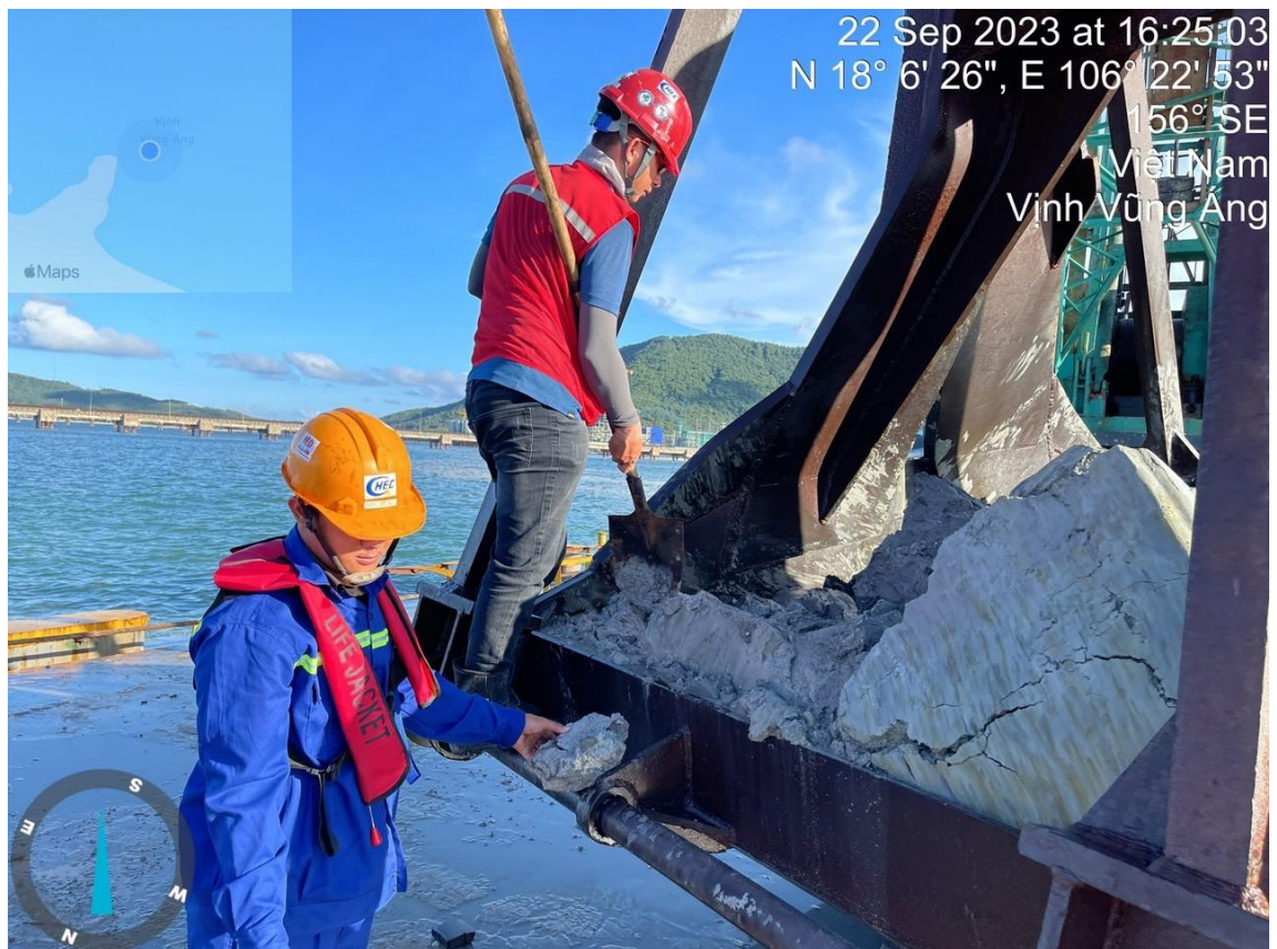
Figure 2.20. Results of the field inspection of dredged material in the intake area on the afternoon of September 22, 2023
