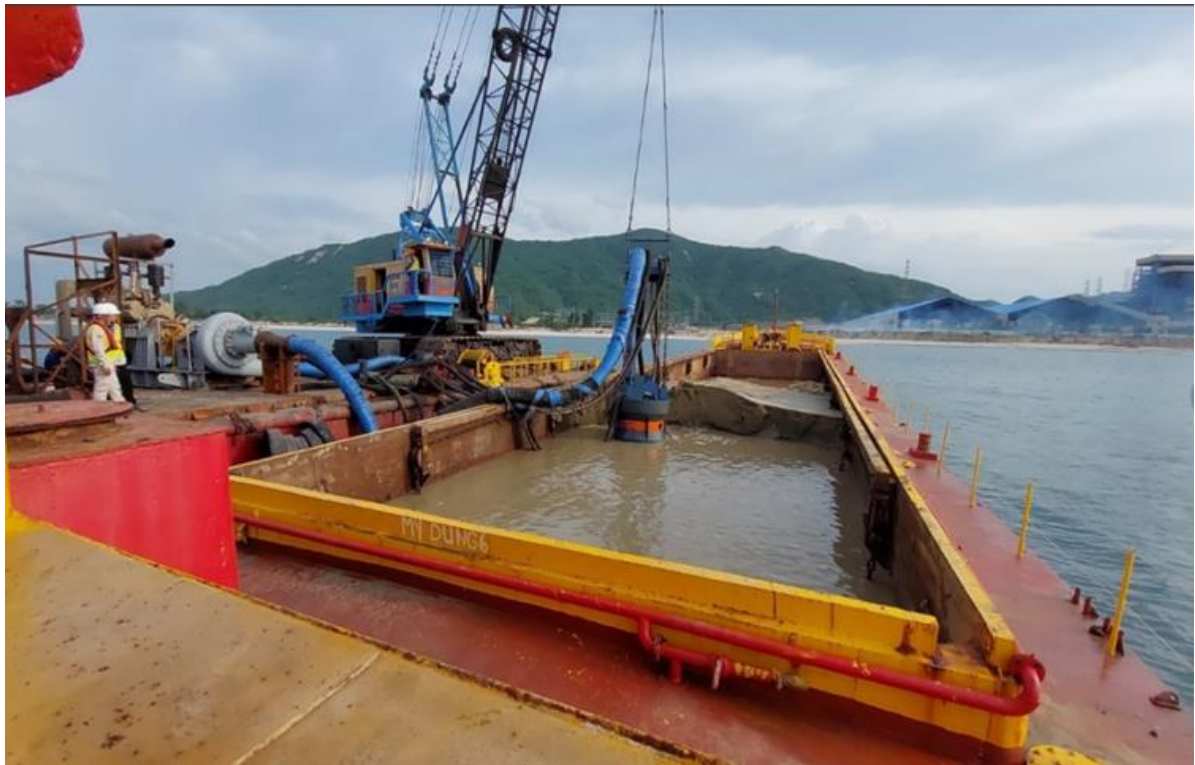
Figure 1.16 Illustration of the transport route of dredged materials from the dredging area to the pumping stations (about 12km)
