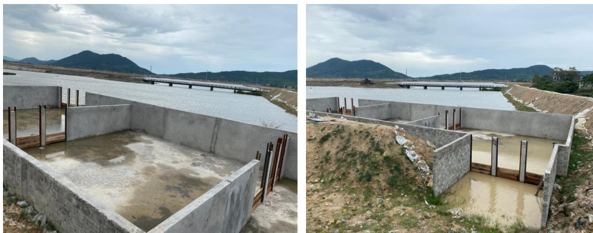
Figure 3.38 Three-stage settling tank for treating runoff water from the containment area
