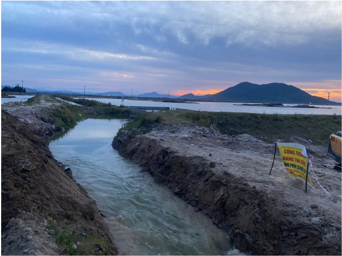
Figure 3.39 Open channel receiving water after the settling tank.
