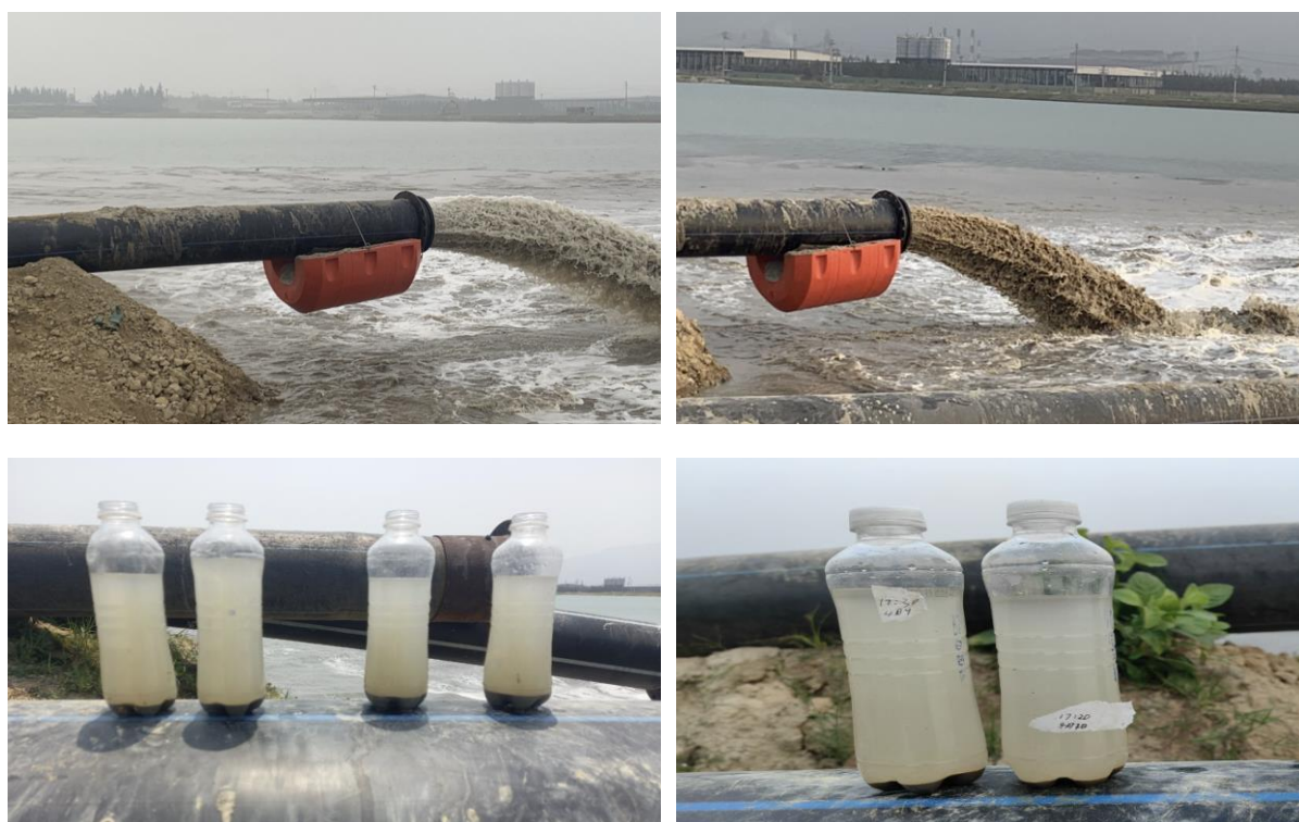
Figure 1.6 The dredged material content in the mixture pumped to the disposal site is less than 5%, resulting in very low work efficiency (water sample taken from the pipe pumping into the disposal site).
